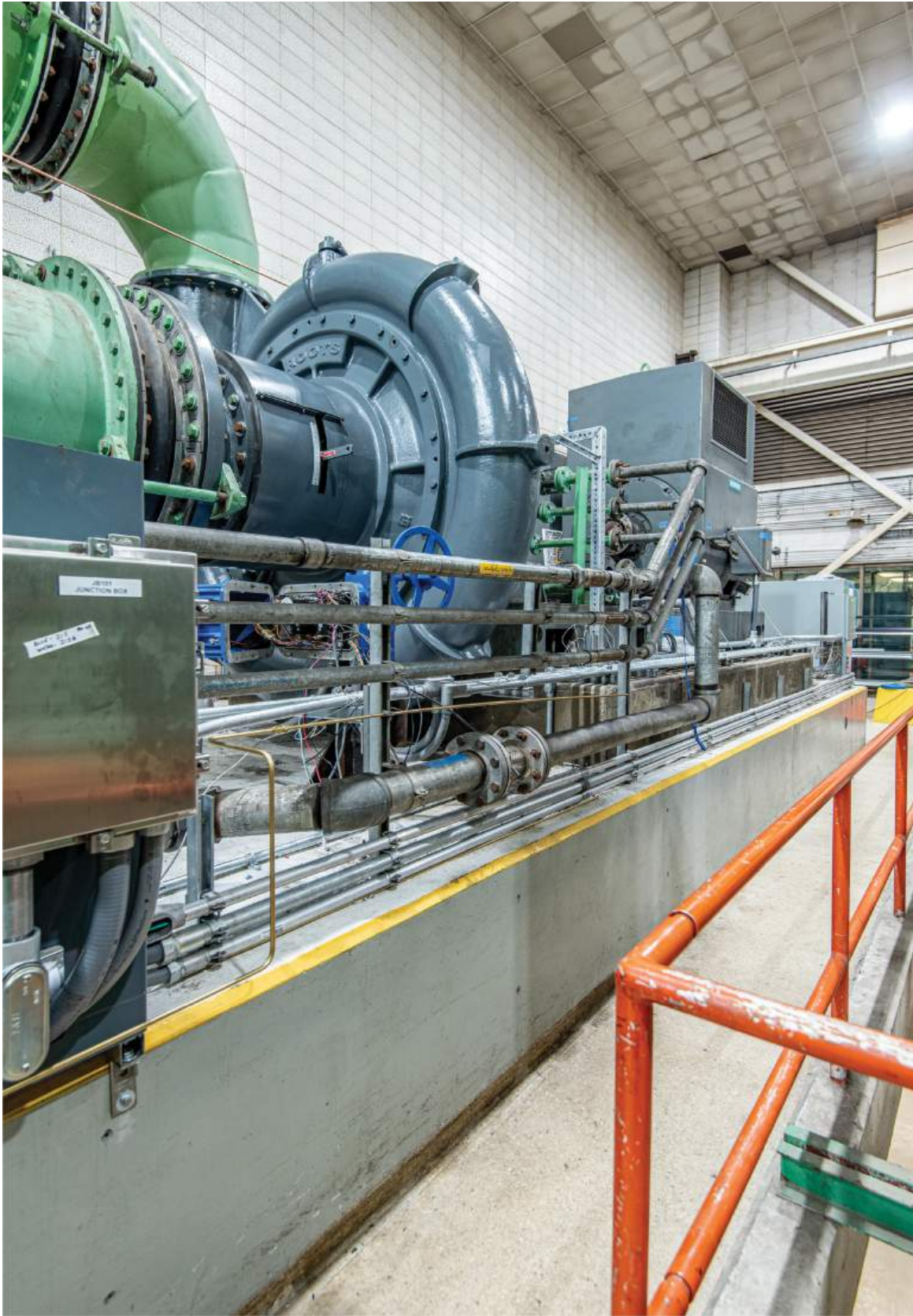
Figure 1-5: Blower 2 – 1 st Floor of Blower Building.
