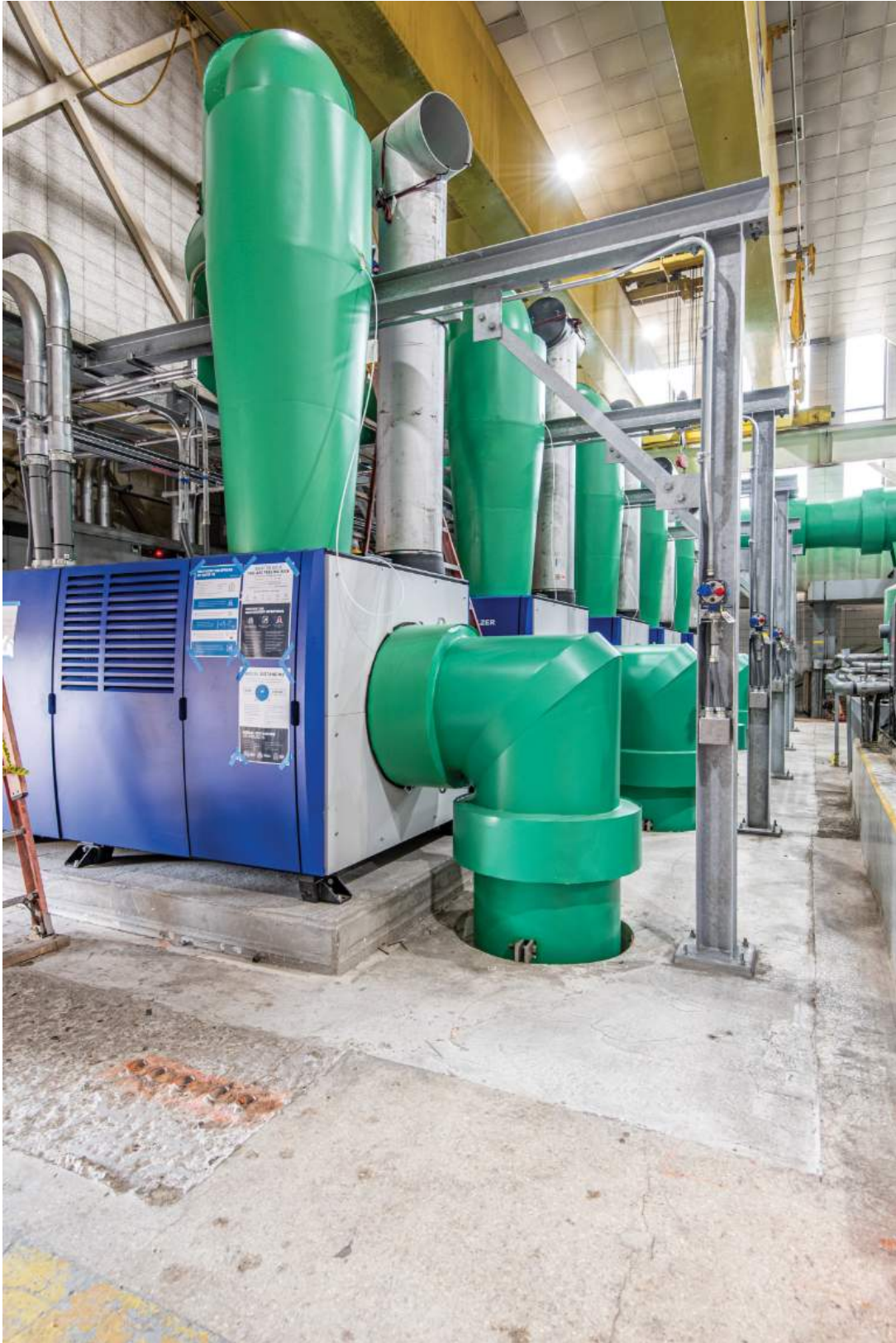
Figure 1-3: Turbo Blowers- 1 st Floor of Blower Building.
