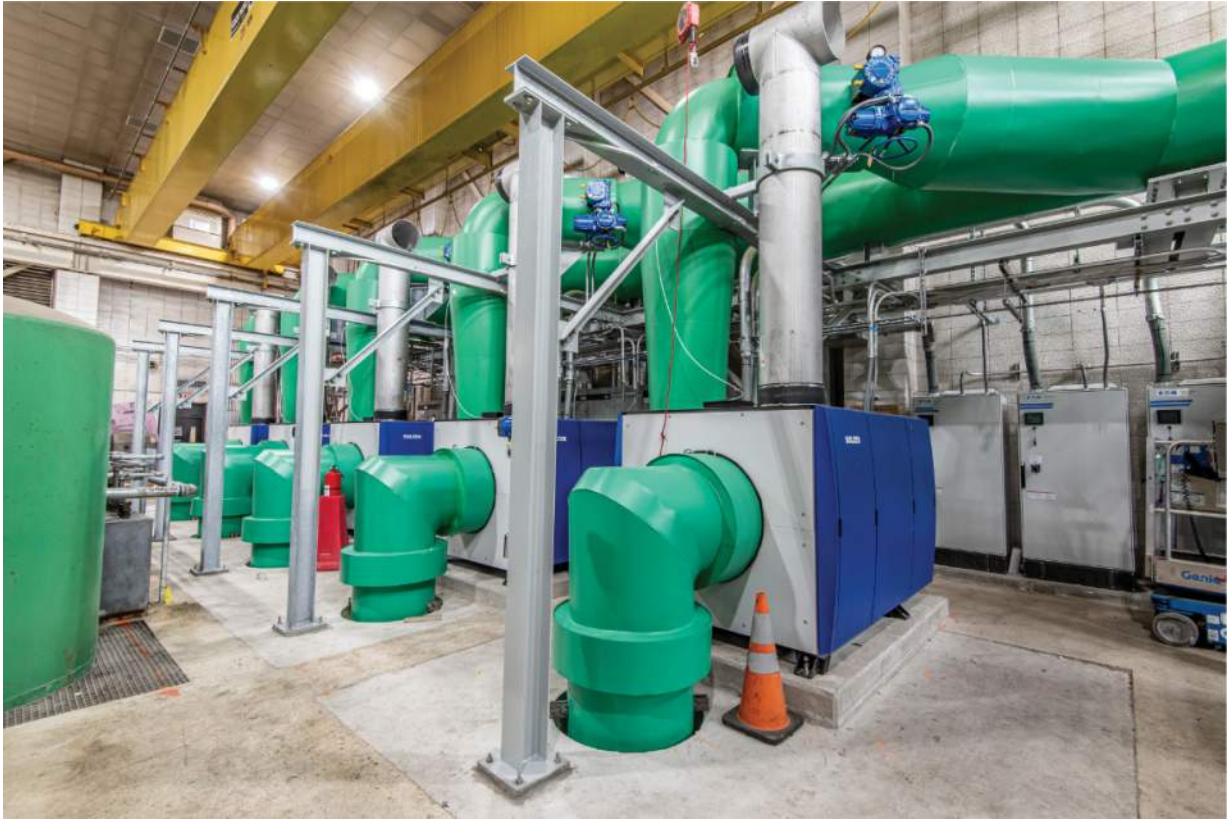
Figure 1-4: Turbo Blowers- 1 st Floor of Blower Building.
