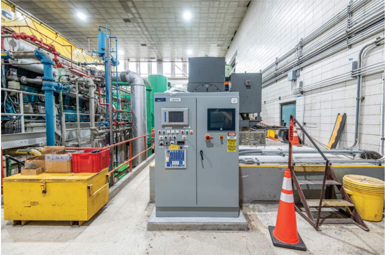
Figure 1-6: Blower 2 and Control panel – 1 st Floor of Blower Building.
